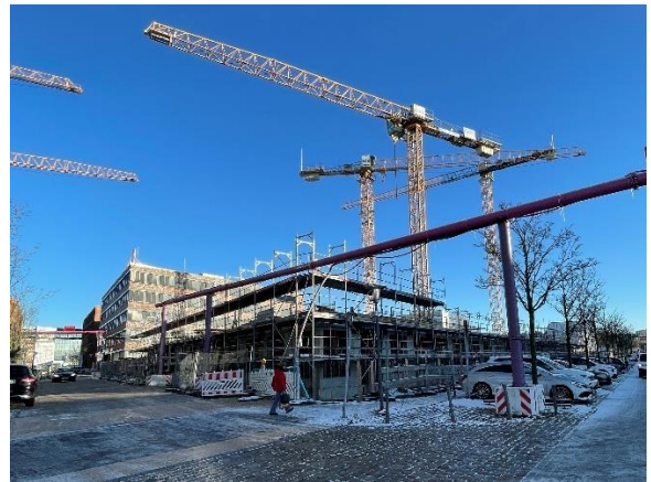
Eastern neighbouring plot, parking entrance closed
