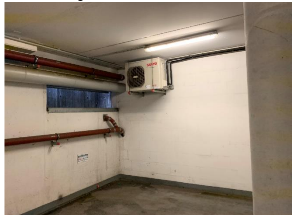
Parking garage, air condition owned by the client
