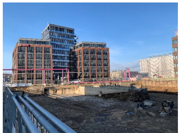
Eastern neighbouring plot, parking entrance closed
